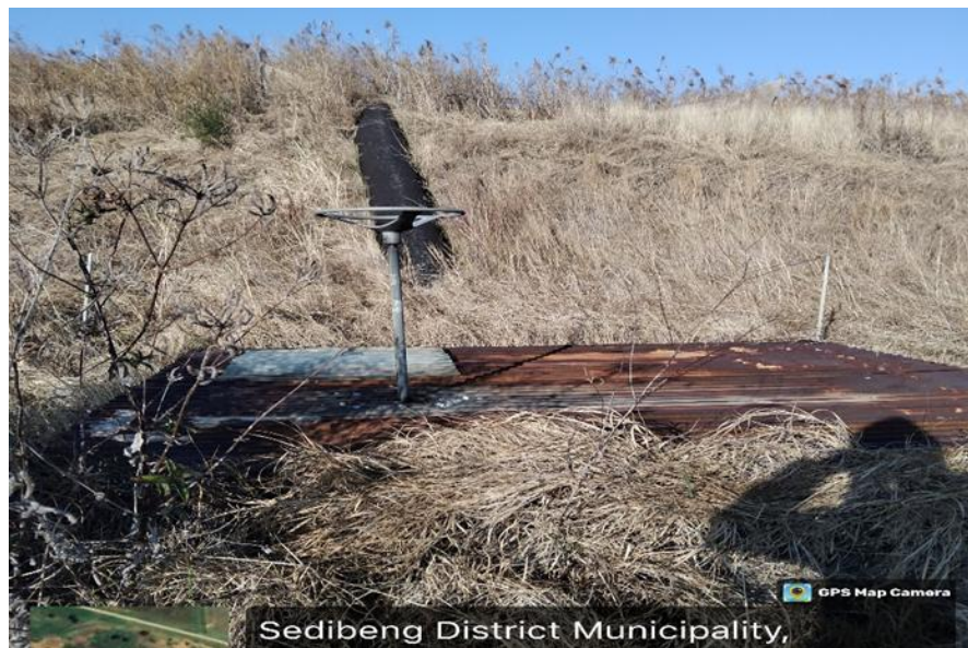
Figure 9: Old pipe system rusted and discarded and located at the far end of the site.
